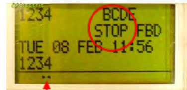
STOP MODE PLC needs to be manually shifted to run mode (see below)
